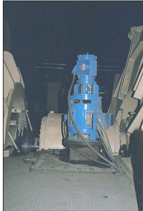
Figure 25: Turbine Turning Gear
