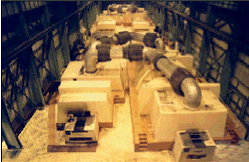
Chernobyl Steam Turbines
